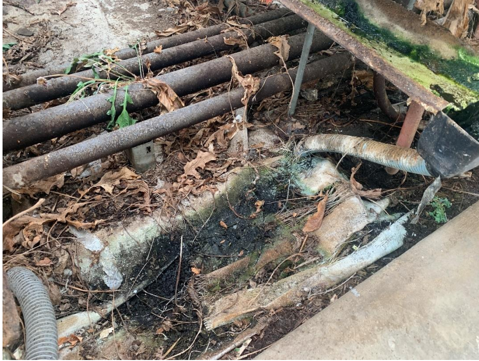
Image 19: Subsurface Irrigation Lines within Greenhouse.
