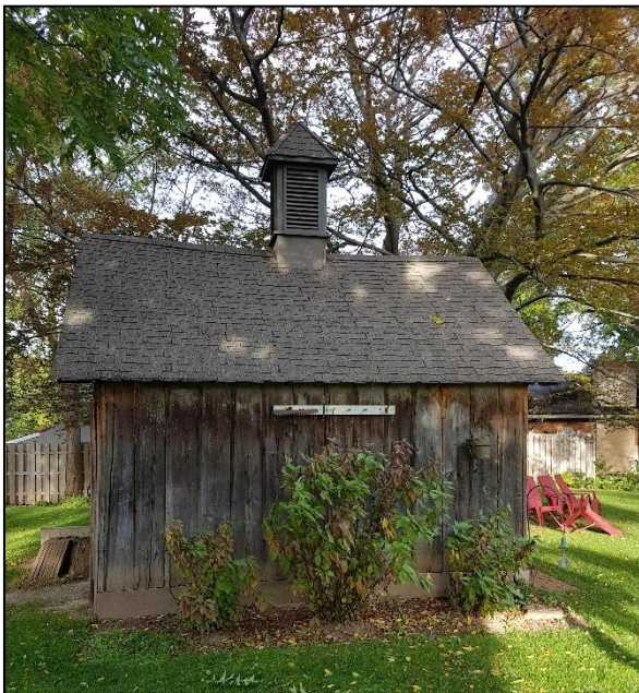
Figure 29: 224 Main Street East, showing east elevation of ice house in rear yard
