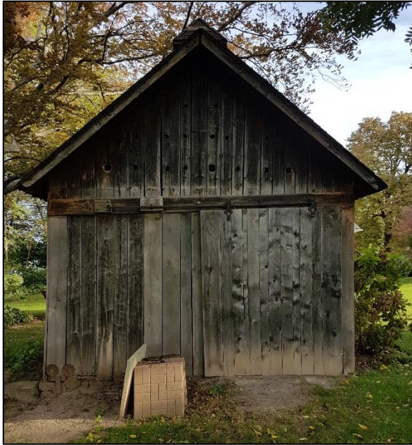
Figure 27: 224 Main Street East, showing south elevation of ice house in rear yard
