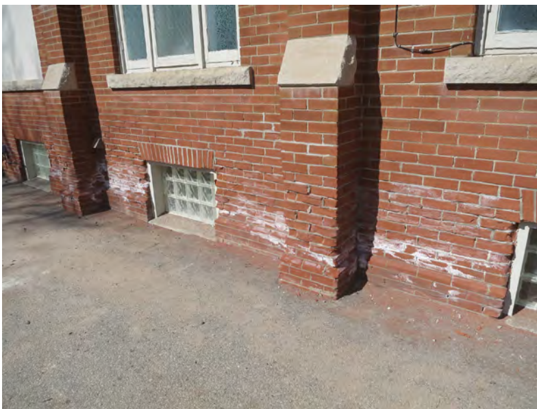
Badly eroded brickwork on east elevation of addition (ERA, 2021).
