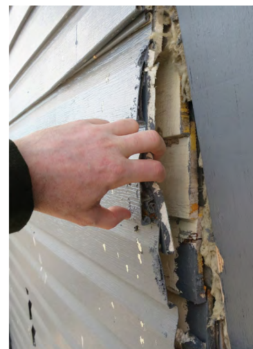
Opening in vinyl siding at rear addition/north elevation revealing wood clapboard siding beneath (ERA, 2021).
