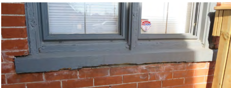
Wood rot in window lug-sill (ERA, 2021).
