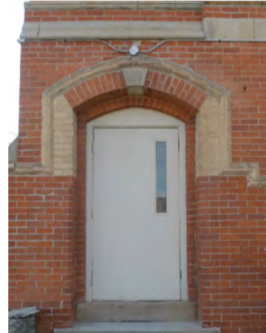
West elevation detail of northern doorway. Remove disused services (ERA, 2021).
