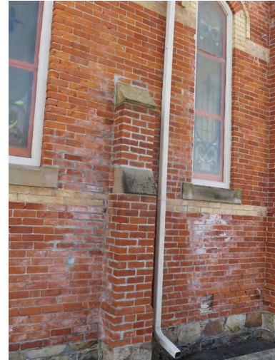
Efflorescence staining on north elevation (ERA, 2021).
