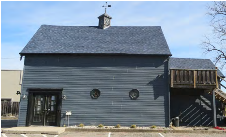
South elevation with uneven vinyl siding installation (ERA, 2021).
