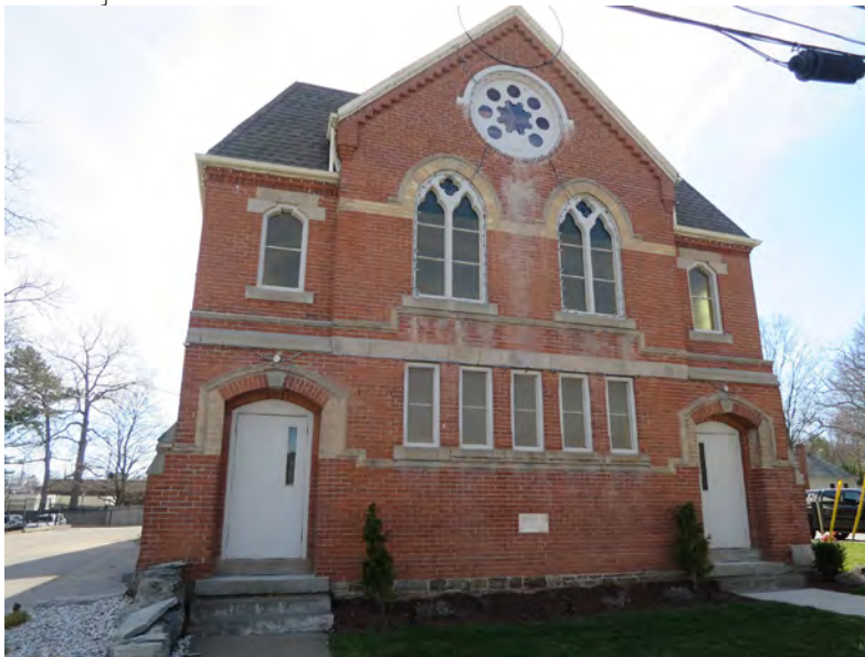
West elevation showing some masonry staining/soiling (ERA, 2021).
