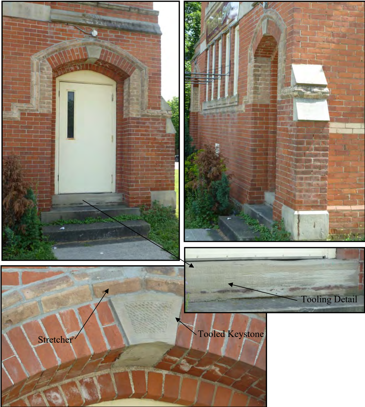
FIGURE 14: Over the doors we see a contrast of colors on the original clay brick arch construction, a soft mortar would have been used to compliment the kiln fired clay brick in a light contrasting color. The arch is constructed with white bricks as the spring of the arch and red clay bricks as the voussoirs, the arch is then completed with a tooled key stone. The completed arch is then traced out with brick. Unlike the arches above the windows the tracing above the doors is done with the stretcher side of the brick. Under the door frame we can see the original tooled cut stone sill.
