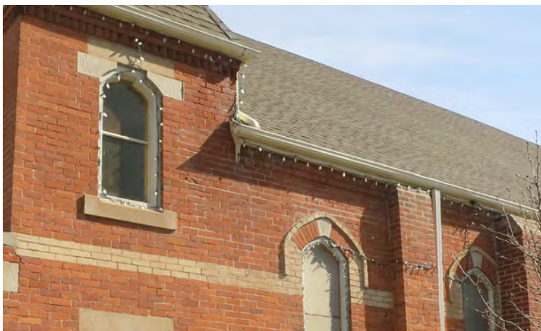
Area of deteriorated/spalled brickwork on south elevation (ERA, 2021).
