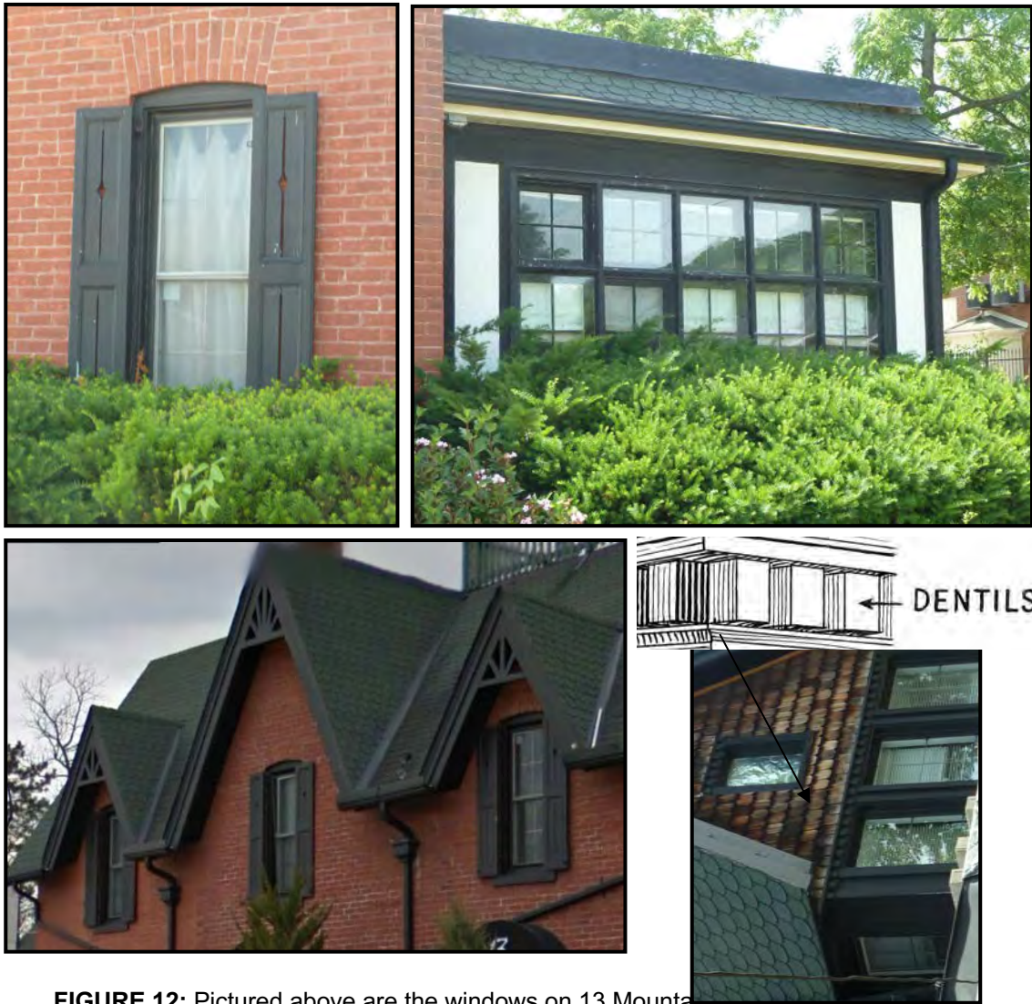
FIGURE 12: Pictured above are the windows on 13 Mountain Street. The wood shutters can be found throughout the exterior facade. The sunroom windows are wood sash windows with 4 over 6 pain division. A detailed peak is shown above with cedar shakes and decorative dentils on wood window surround. Segmental arches can be seen above the original window openings.
