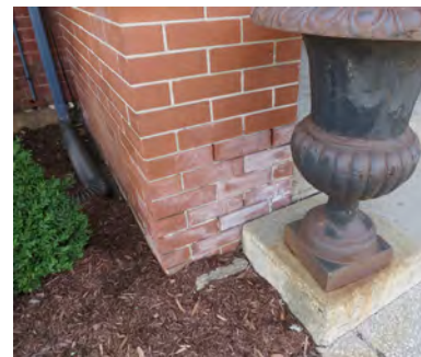
Open mortar joints in brick and stone foundation masonry (ERA, 2021).
