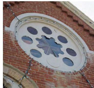
Open joints at perimeter of rose window on west elevation (ERA, 2021).
