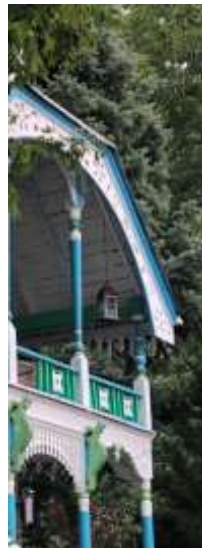
(far left) spindle bracket (middle) hip and gambrel roof, (right) ornate columns, gingerbread (bargeboard) and skirting
