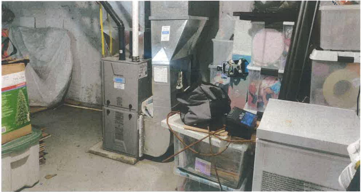
General view of the furnace in the basement of the residential structure at the subject site
