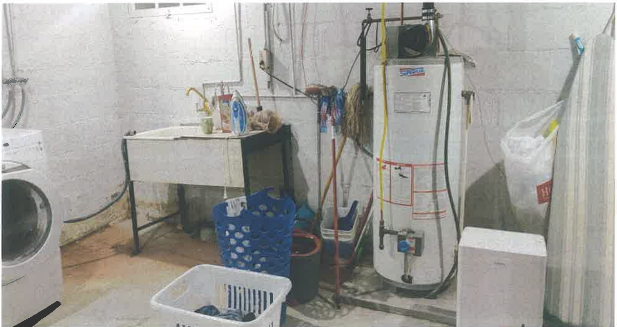
General view of the water heater in the basement of the residential structure at the subject site
