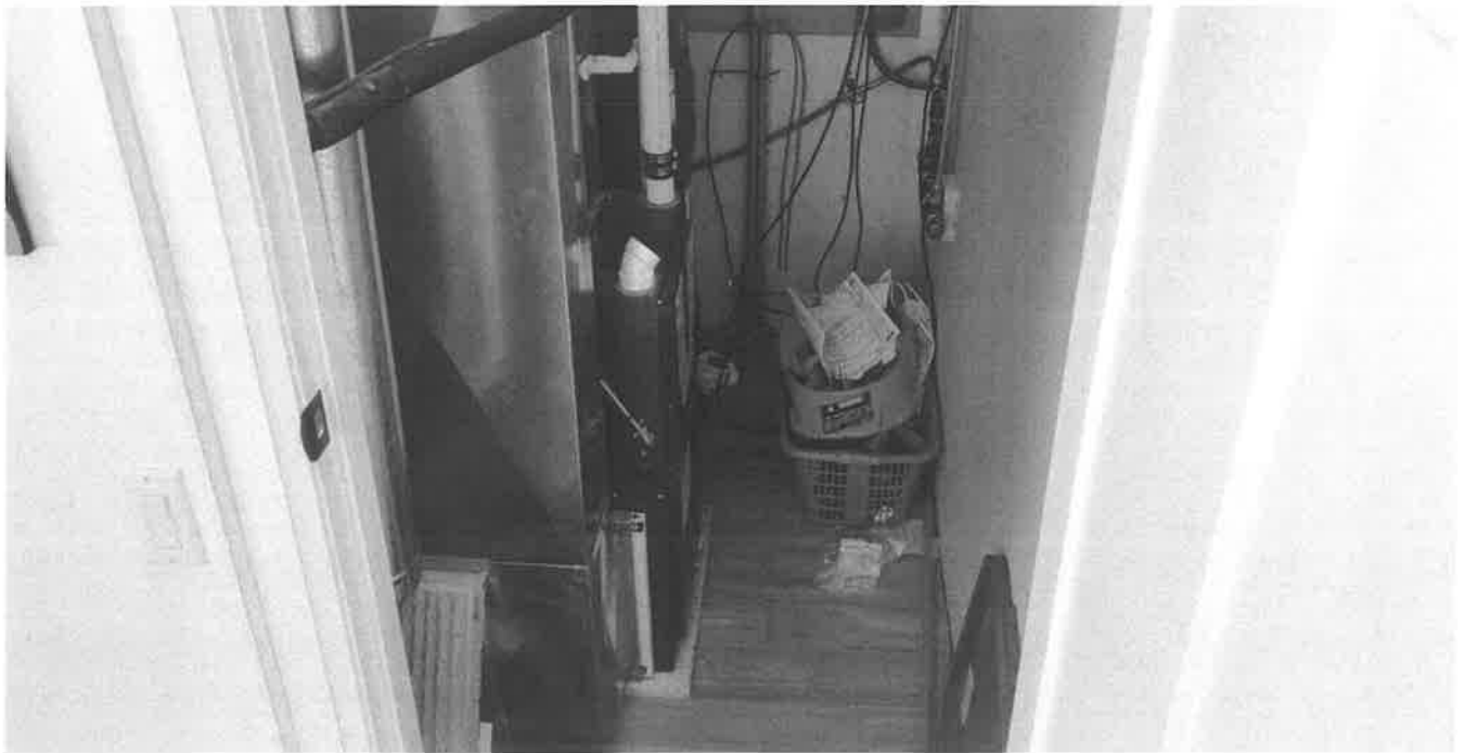
General view of the furnace at pool house at the subject site
