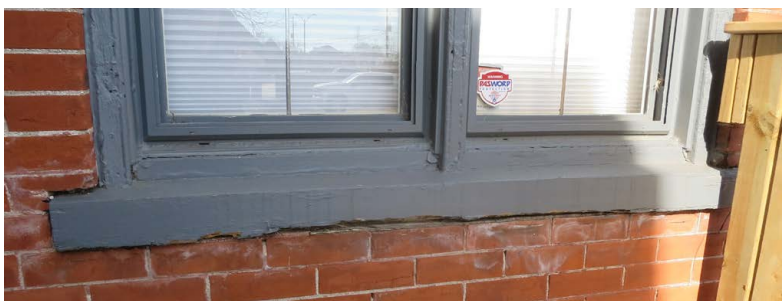
Wood rot in window lug-sill (ERA, 2021).
