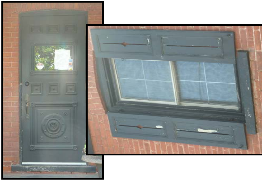
FIGURE 13: Pictured above are the detailed wood shutters and wood door. The detailed wood work can be seen throughout 13 Mountain Street.
