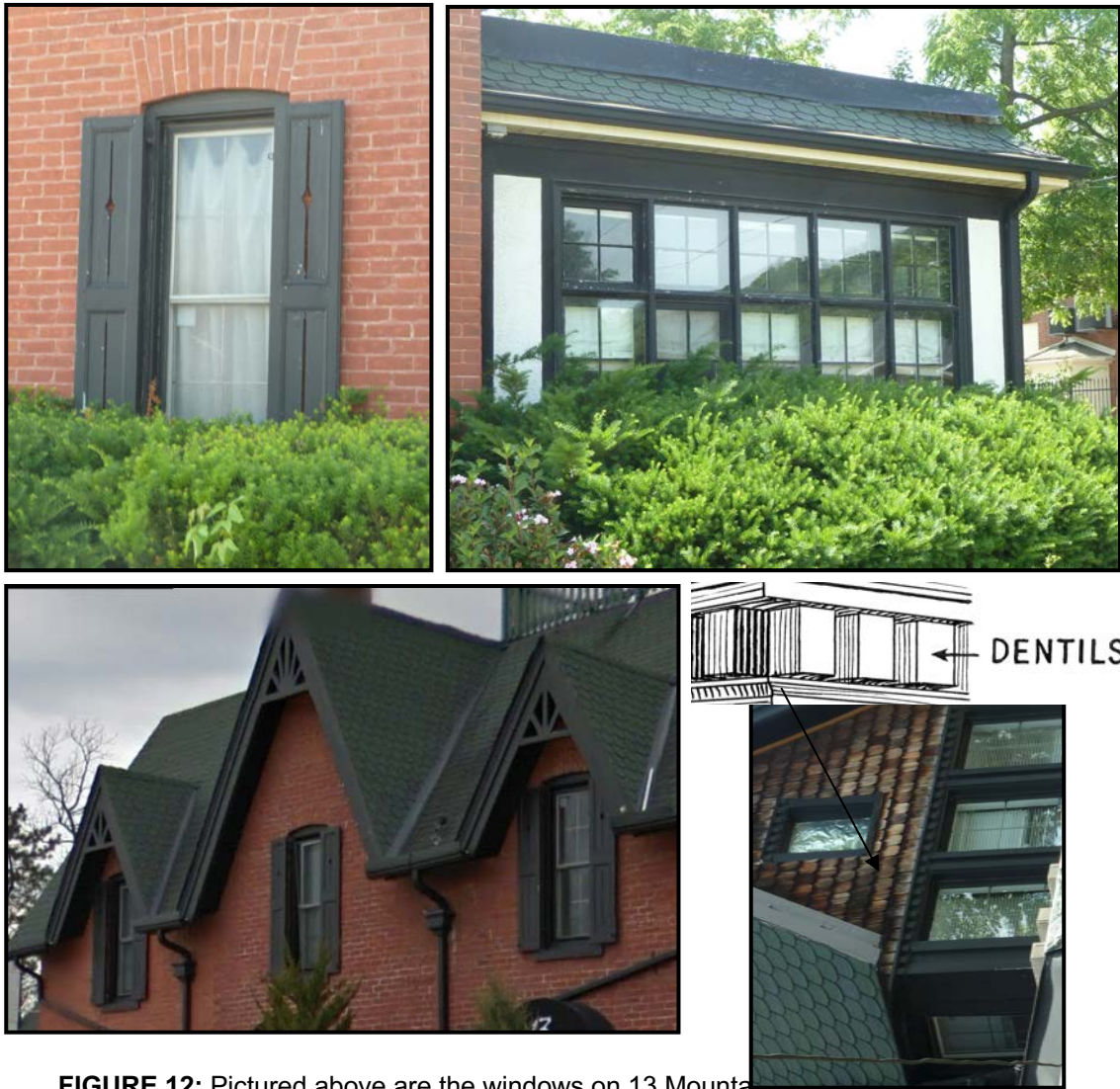
FIGURE 12: Pictured above are the windows on 13 Mountain Street. The wood shutters can be found throughout the exterior facade. The sunroom windows are wood sash windows with 4 over 6 pane division. A detailed peak is shown above with cedar shakes and decorative dentils on wood window surround. Segmental arches can be seen above the original window openings.
