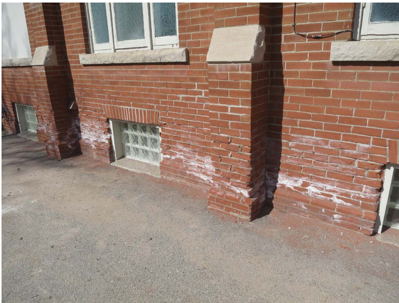
Badly eroded brickwork on east elevation of addition (ERA, 2021).
