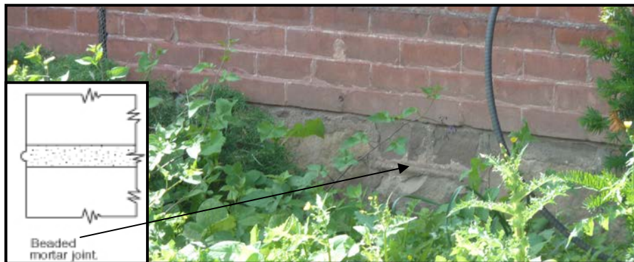
FIGURE 7: 13 Mountain Street is a red clay brick structure built on a stone foundation. The original foundation was arranged in a coursed layout using cut stone and a lime based mortar. The foundation mortar shown above has a beaded mortar joint. The face of the cut stone was left with a quarried finish.
