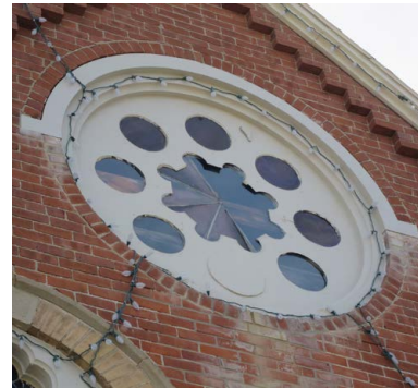
Open joints at perimeter of rose window on west elevation (ERA, 2021).
