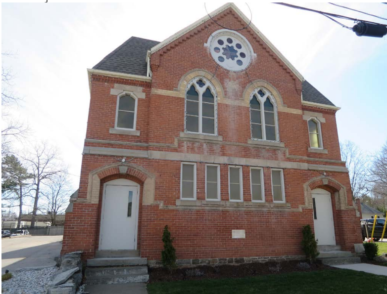
West elevation showing some masonry staining/soiling (ERA, 2021).
