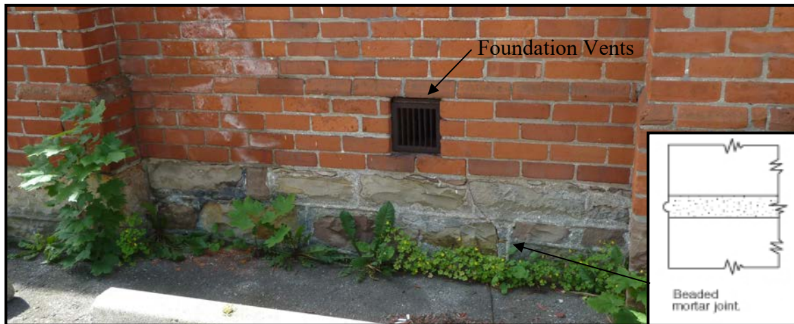
FIGURE 11: 19 Elm Street is a clay brick structure built on a stone foundation. The original foundation was arranged in a coursed layout with a cut stone and lime based mortar. The foundation mortar shown above has a beaded mortar joint. The face of the cut stone was left with a quarried finish. Pictured above you can also see the foundation vents which were used to keep the air circulating in the basement to prevent the spread mold and mildew in the summer months.
