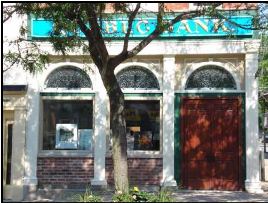
Figure 7: The completed façade restoration works for the building seen in Figure 5. These restoration works represent good practice.
