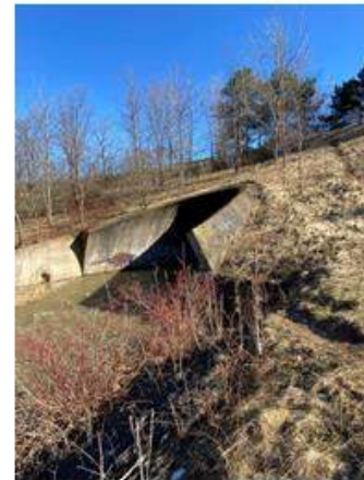
Forty Mile Creek tunnel @ South Service Road. Evidence of use for walking.
