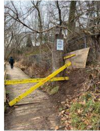
Existing signage marking the bridge as closed
